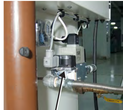
Gas Pressure Switch on multiblock gas valve
