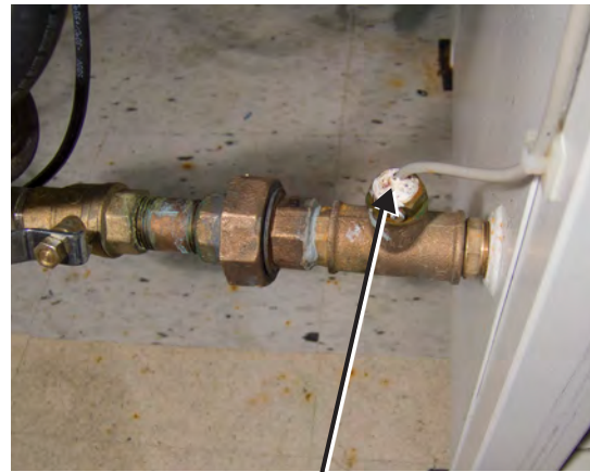
Buffer tank return line temperature sensor mounted near rear wall of microCHP cabinet
