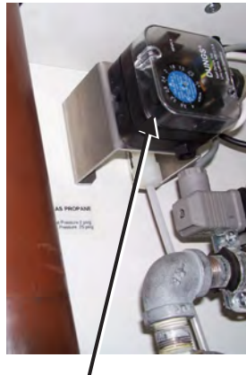
Differential Pressure Switch mounted on back of microCHP cabinet
